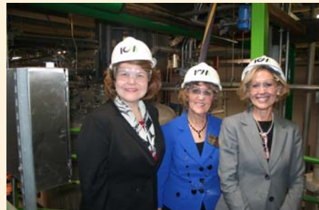
Administrator Judy Canales is joined by Missouri State Director, Anita J. (Jamie) Dunning and Kansas State Director, Patty Clark as they tour the ICM-Lifeline Foods Cellulosic Ethanol Pilot Plant in St. Joseph, Missouri.
